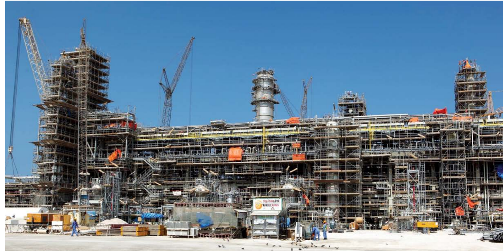
A section of the under construction Laffan Refinery 2. Laffan Refinery 2 will house the new Water Recycling Facility, which will also serve Laffan Refinery 1 already in operation.
